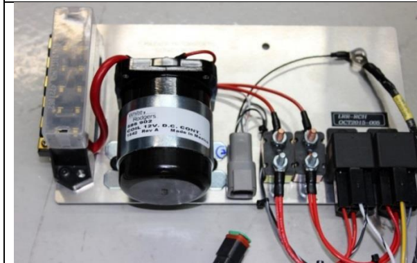
Power Distribution Panel – A 0000-08-5052
