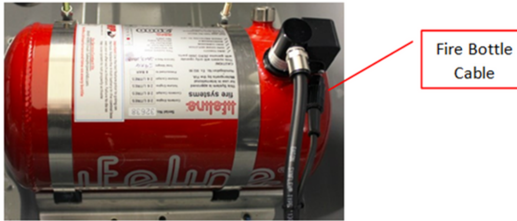
Figure 3. Fire Bottle Cable, Trunk.
