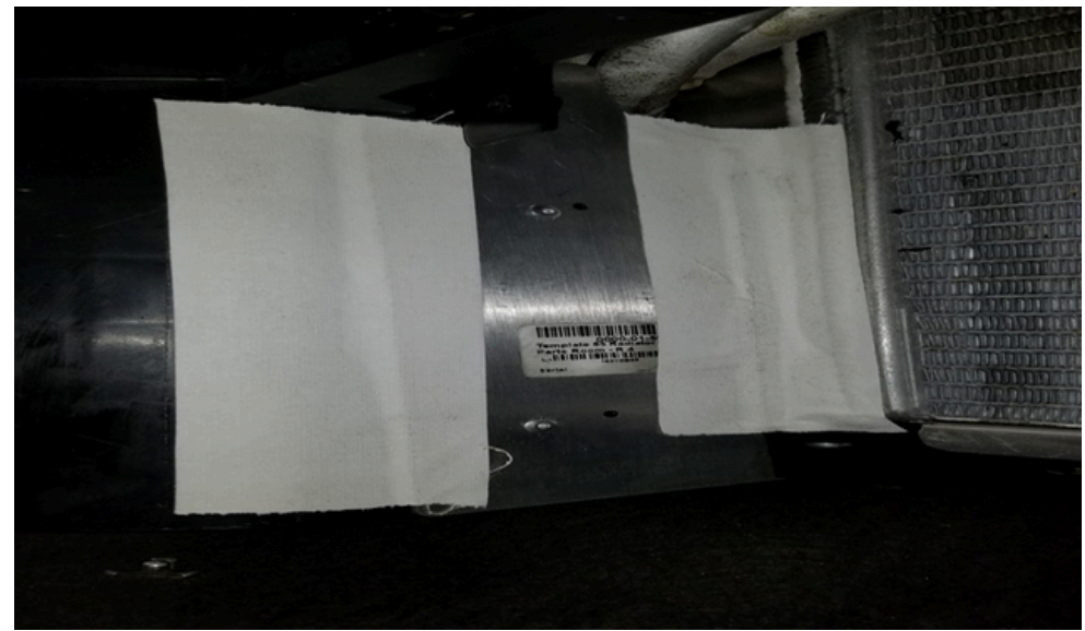
Use of White Gaffer Tape Required Taping of Duct Work is open. Tape Up Gaps and Seams in Radiator Ducting
