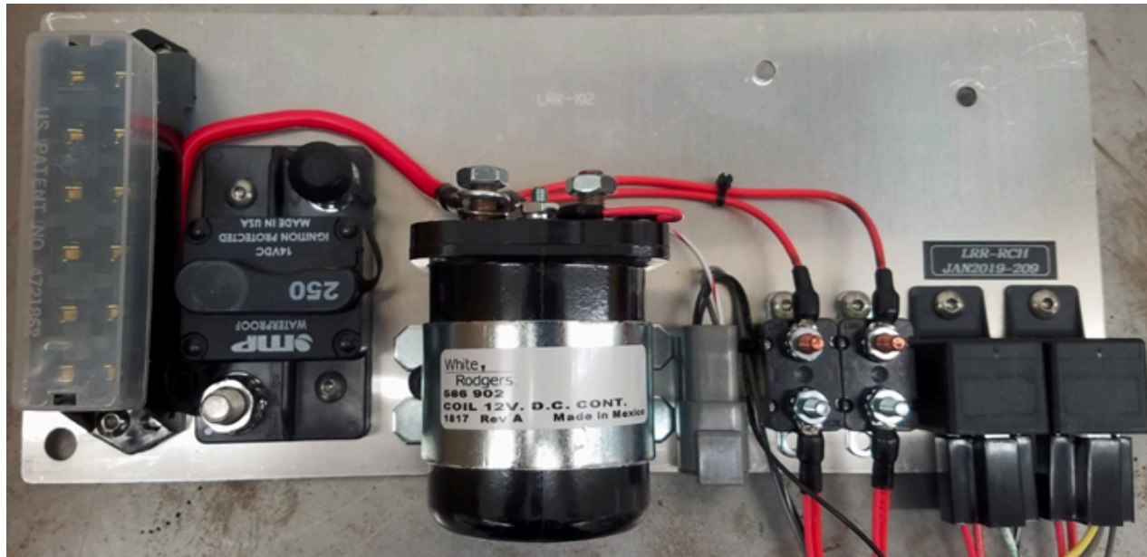
Figure 7: Power Distribution Panel (Trunk)
